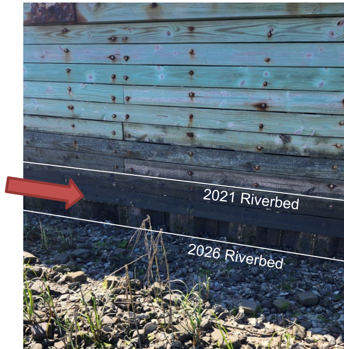
Figure 3. Exposed Seawall Toe in Area of Riverbed Soil Erosion
