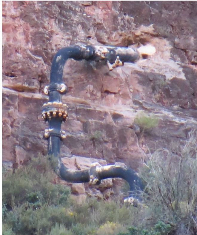
Figure 10: Existing waterline exiting a borehole below the South Rim along the Bright Angel Trail
