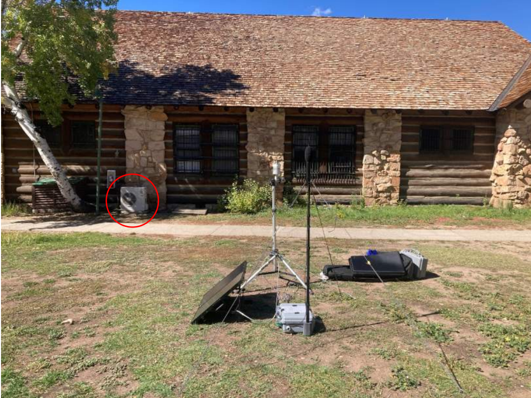
Grand Lodge Site Looking North Towards Cabins (top) and East Toward Main Building (bottom) – Note Chiller Circled in East View
