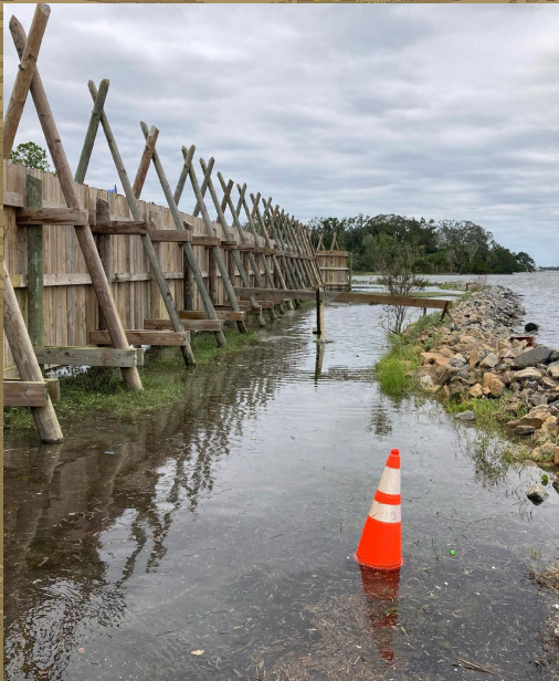
Flooding at Fort Caroline
