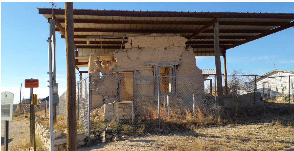
Figure 42. Ruins of the J.D. Holiday Sutler Store, showing a partially collapsed adobe structure enclosed by a chain-link fence surrounding the site
