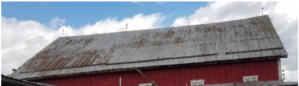
The south slope of the barn gable roof is covered with modern corrugated metal panel. Note the deteriorated paint. Photo: HPTC, 06/21/17.
