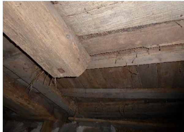
J20 has been cut and bolted to the floor board above. Photo: HPTC, 06/21/17.
