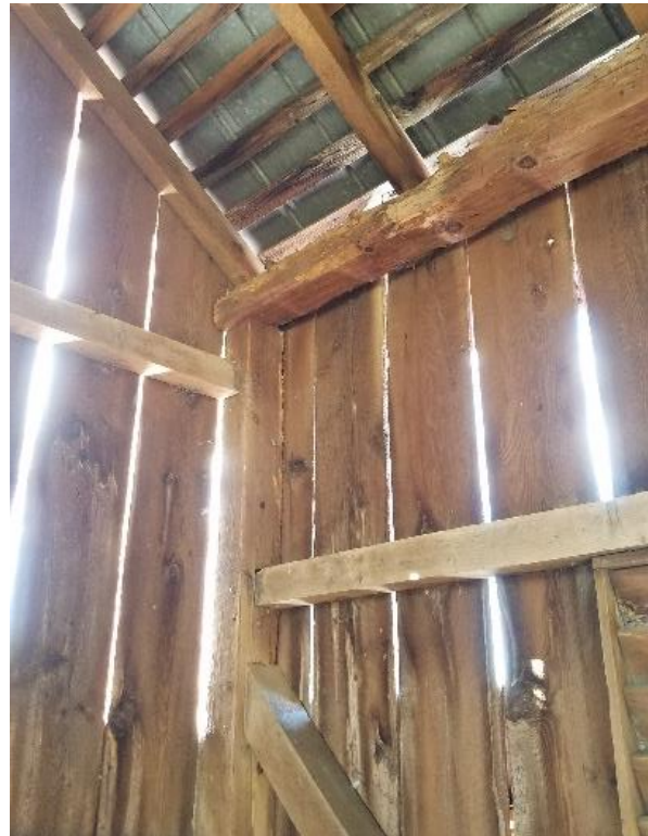
Right: Insect damage on the southeast corner and roof plate of the south elevation. Photo: HPTC, 06/21/17.
