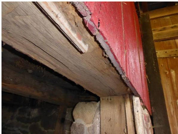
The east elevation sill exposed at the window opening. Photo: HPTC, 06/21/17.
