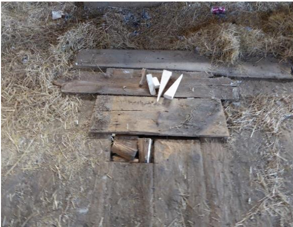
Broken and patched floor in the threshing bay. Photo: HPTC, 06/21/17.
