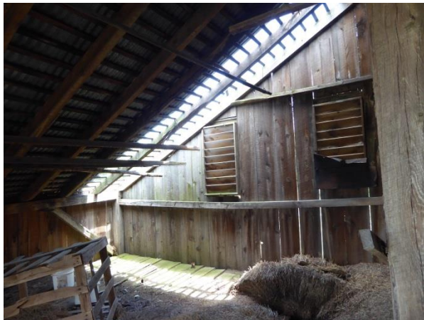
The interior elevation of the outshed granary's east wall. Damage has occurred to the structural members due to the missing roof covering. Photo: HTPC, 06/21/17.
