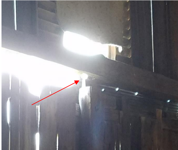
Tenon of the center west wall post is removed from its mortise as the wall is pulled down by failing foundations and framing below. Photo: HPTC, 06/21/17.
