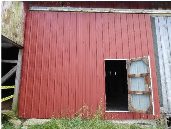
D101 is a large sliding modern barn door with inset man door. Photo: HPTC, 06/21/17.
