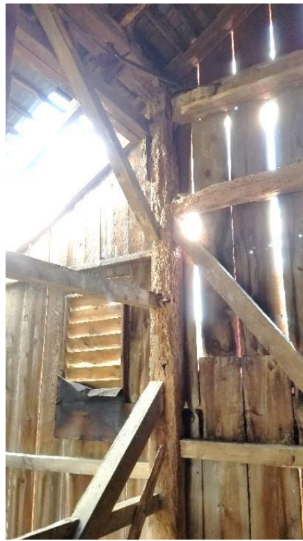
Significant rot and insect damage on the northeast end post. Photo: HPTC, 06/21/17.
