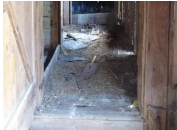
The flooring in the interior granary is deteriorated. Photo: HPTC, 06/21/17.
