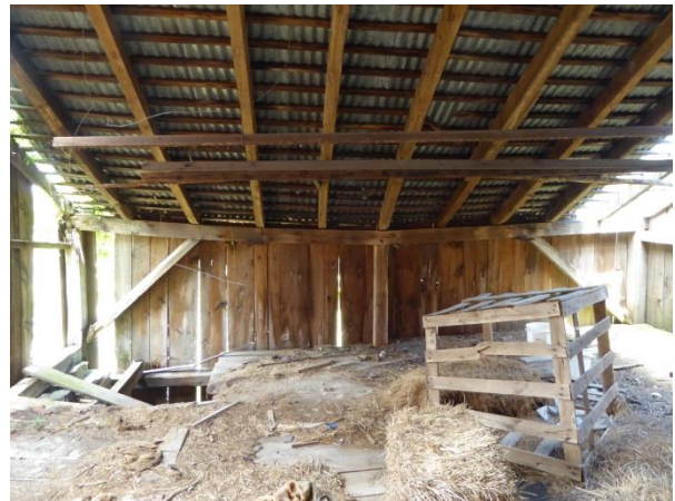
The interior elevation of the outshed granary's north wall. Damage has occurred to the structural members due to damage to the foundation wall below. Photo: HTPC, 06/21/17.
