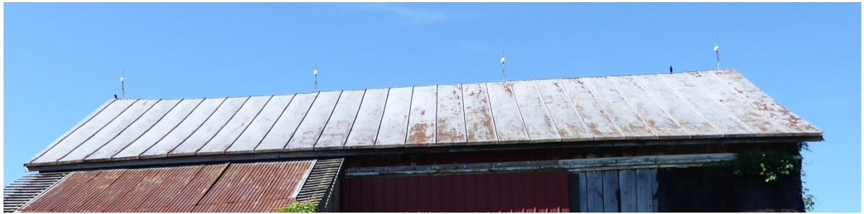
The north slope of the barn gable roof is covered with historic standing-seam metal. Note the deteriorated paint. Photo: HPTC, 06/20/17.
