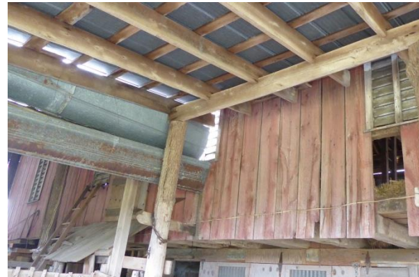
A missing piece of siding on the south elevation, under the later garage addition. Photo: HPTC, 06/21/17.
