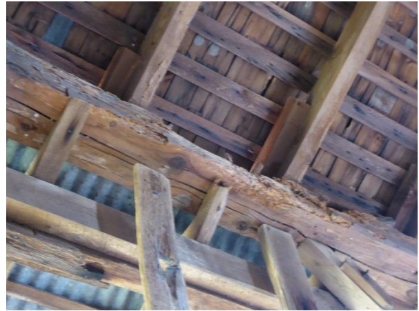
The roof plate of the north elevation has insect damage at its eastern end. Photo: HPTC, 06/21/17.
