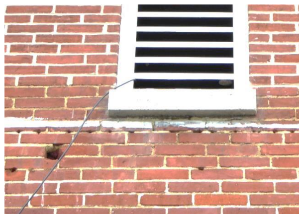
South elevation detail. Note holes below white ghost line, likely where the roof of a non-extant addition was connected, and void at bottom left, possibly to pocket a framing component into masonry. Photo: HPTC, 06/07/17.
