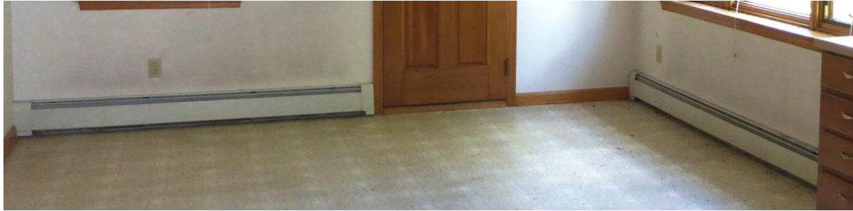
Hot-water baseboard radiators, Room 102. Photo: HPTC, 06/08/17.
