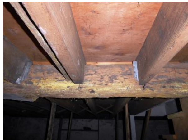
Some galvanized joist hangers have been added between the joists and the summer beam. Note extensive rot and mold, joist sistering, and modern joist hangers. Photo: HPTC, 06/08/17.
