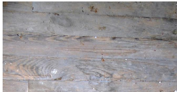
Historic wood flooring in Attic (Room 301) is a CDF. Photo: HPTC, 06/08/17.
