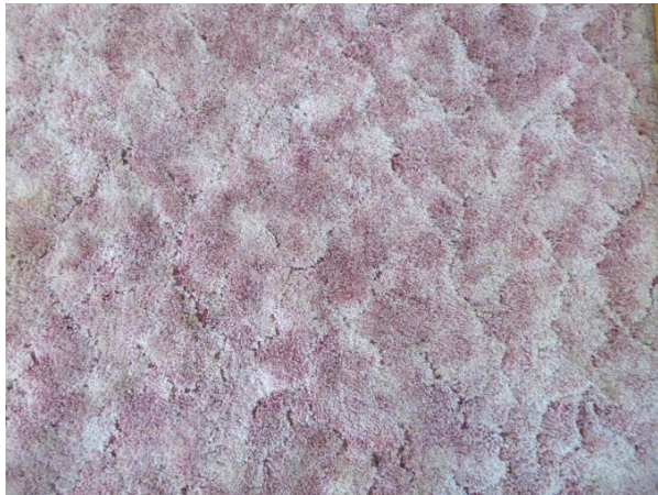
The sunroom, living room, dining room, and bedrooms have carpet, which is not a CDF. Photo: HPTC, 06/08/17.
