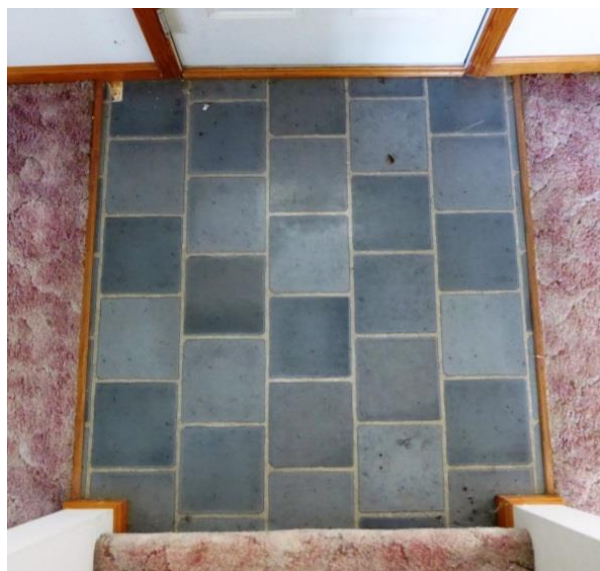
Sheet linoleum between Rooms 104 and 105 mimics natural stone tile. Note area of damage (upper left). Photo: HPTC, 06/08/17.
