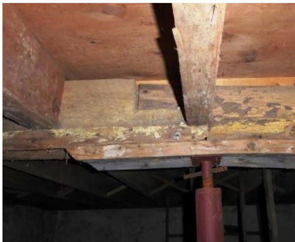
The half lap joint of the two timbers of the summer beam. Both lengths of the beam are extensively deteriorated. Photo: HPTC, 06/08/17.
