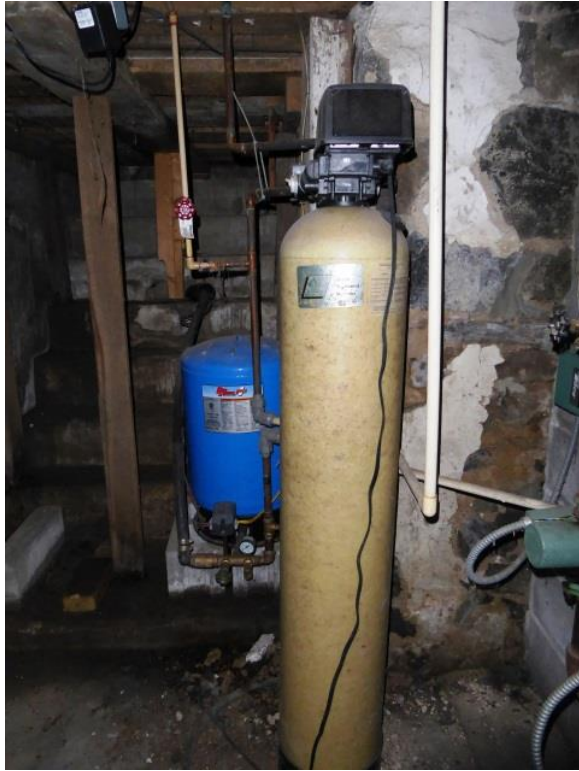
Left: "Pro-Source Plus Steel Pressure Tank" (blue) and "Aqua Treatment Service, Inc. Water Treatment Systems AF163-2D" (tan). Photo: HPTC, 06/08/17.
