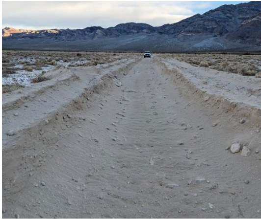
Flood-damaged narrow roadway at Eureka Valley. NPS/Jeremy Stoltzfus
