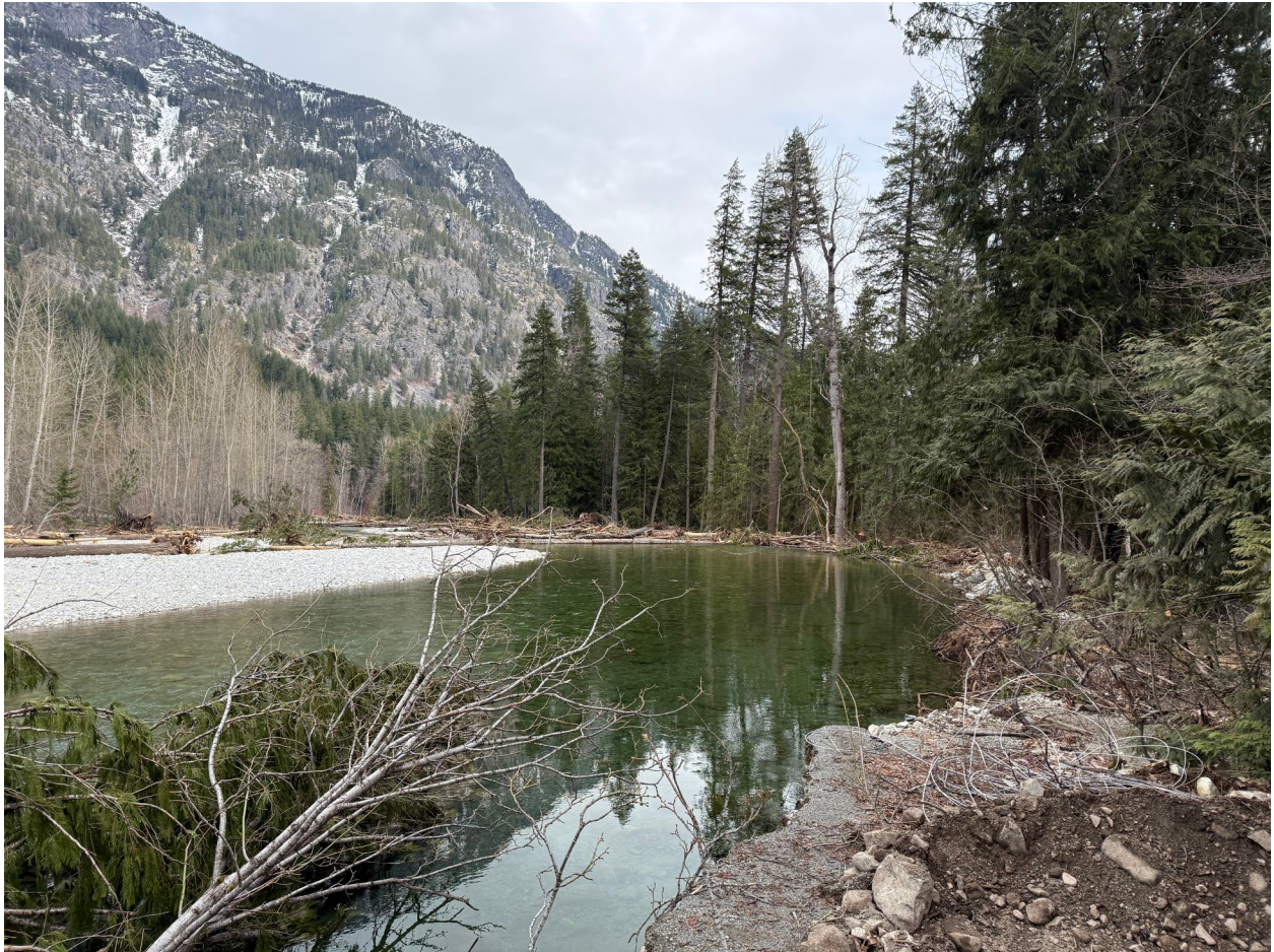
Figure 7. View east from the western washout of Company Creek Road on 3/9/2026 prior to emergency road construction. West end of the Chelan County Road segment will be constructed from this point forward (east) into river, then curve right to connect with the NPS temporary road.
