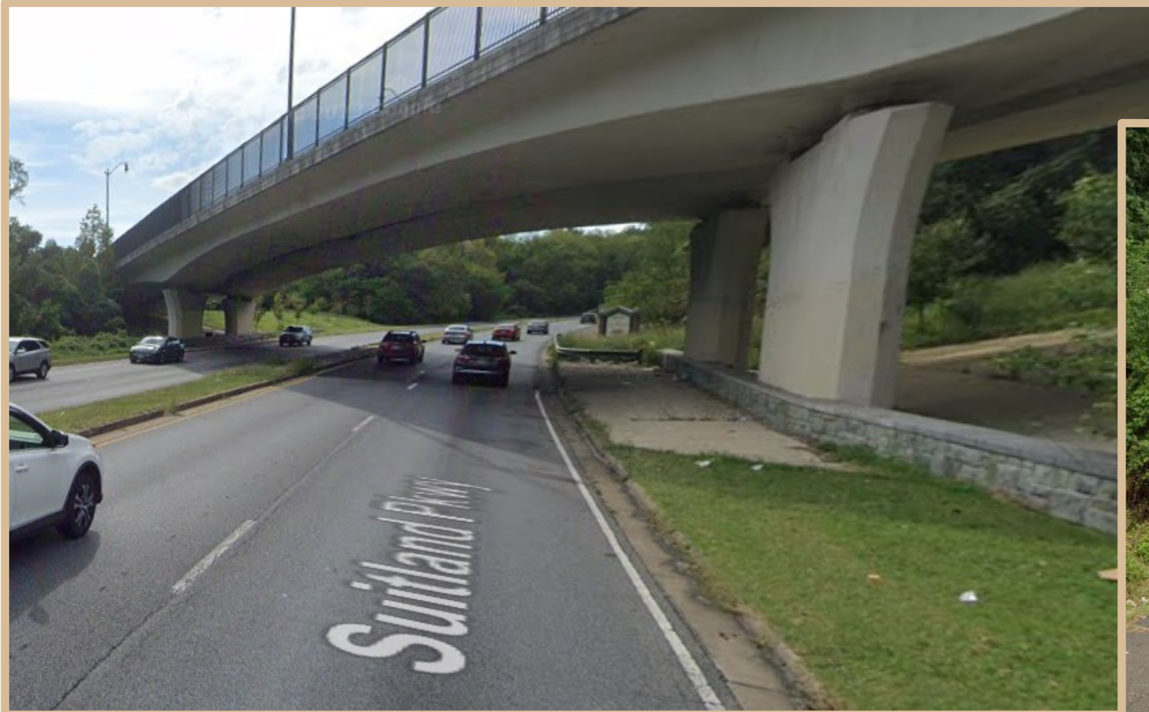
Above: View of westbound Suitland Parkway at Southern Ave. overpass, near DC/MD border and existing trail terminus.
